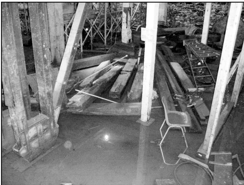
The flooded basement after the water level had dropped about eight feet. High water on Rock Creek
