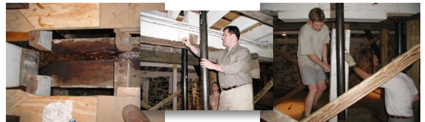
Images of recent work on the support beams at the Mill. Left: Completed work on the main beam showing steel rods set in epoxy. Engineer Brandon Rossetti (center) inspecting the beam after column removal. At right, Steve Ortado and assistant John Waters removing the old column supporting the main beam.
