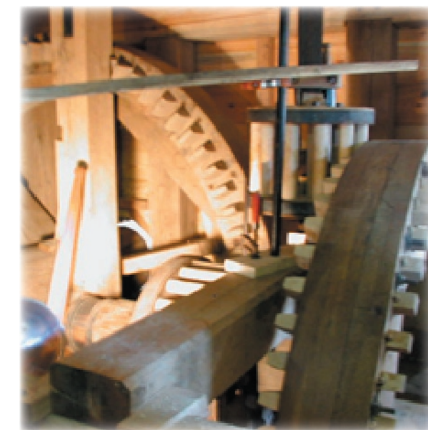
The Grist Mill at Mount Vernon is nearing completion of an extensive restoration. FOPM Board members visited the mill on February 28 to compare work there and envision a similar future for Peirce Mill.
